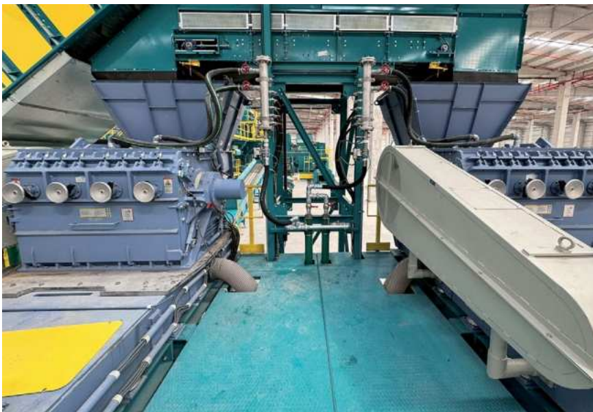
As a central process stage within the PET washing line, the hot wash system in batch design enables controlled temperature management and defined dwell times for efficient removal of labels, adhesives and organic residues
