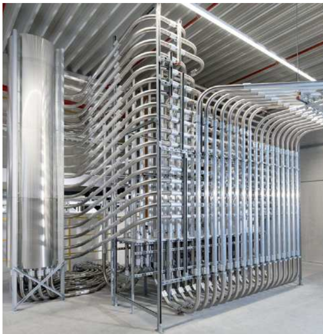
Two fully automatic Metrolink coupling stations draw material from 24 silos and distribute it to the extruders via almost 2,000 metres of piping (Source: motan)
