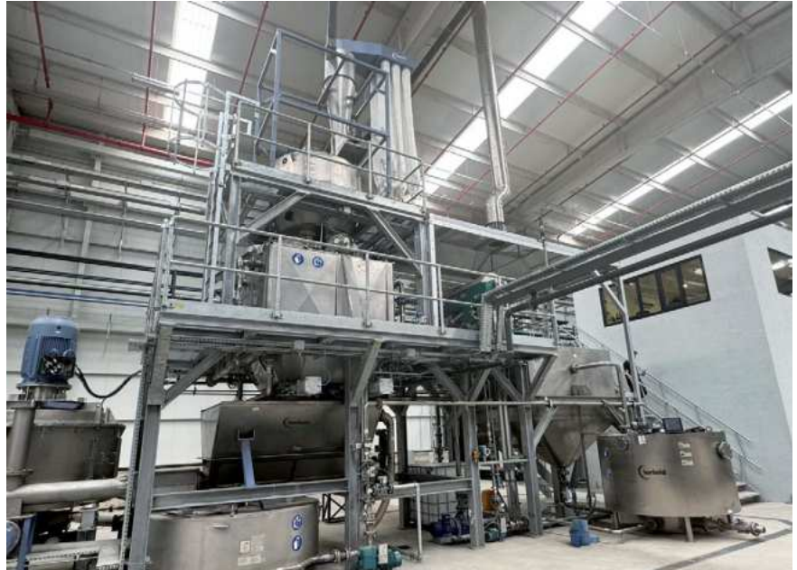
The two SMS forced feeding granulators installed in the first line ensure uniform flake size and stable material intake, creating ideal conditions for downstream washing and density separation processes (Photos: Herbold Meckesheim, Germany)
